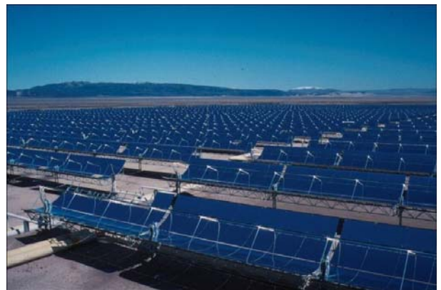
Parabolic trough collector field for the solar thermal power plants in Kramer Junction, California
