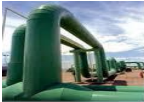
Figure 9: Pipeline for hydrogen delivery
