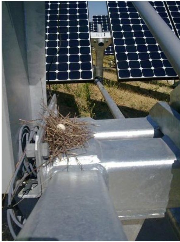
Figure 5: A Nest on Solar Field
